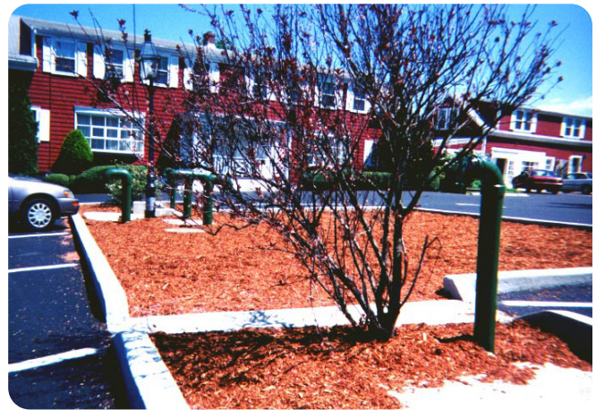
Smith & Loveless provided the Modular FAST® wastewater treatment system (top) to a historic hotel to help the facility maintain its seasonal variations of flow based on tourism. Placing the system underneath the parking lot (below), keeps the establishment aesthetically pleasing.
