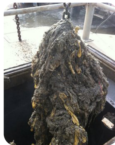
Submersible pump being pulled for maintenance will require cleaning first
