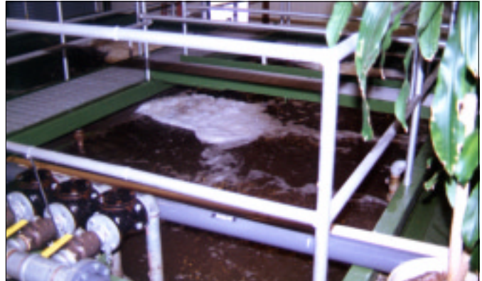
FAST media was added to an existing aeration basin, creating a fixed-film, stable process for effective nitrogen reduction.
