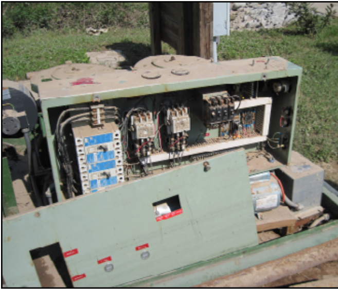
The control panel of this pump station has been dried out and the pumps put back online after it was submerged in the May 1-2, 2010 flooding that occurred in Middle Tennessee.
