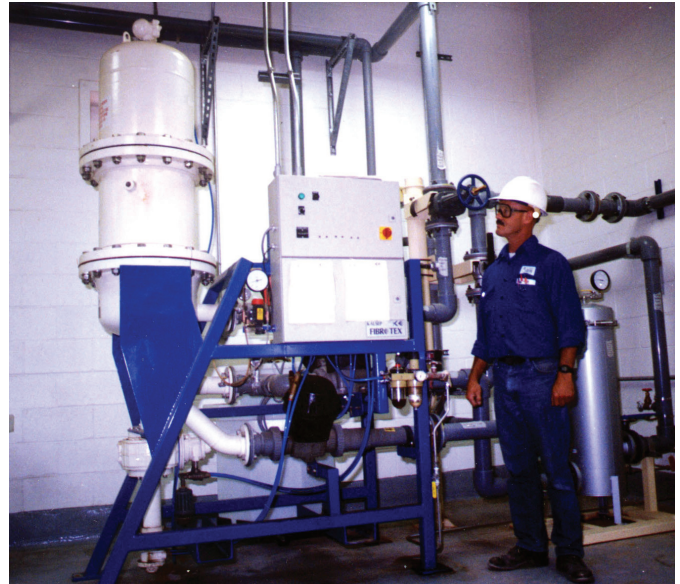
The FIBROTEX® fine filtration system serves as excellent pre-filtration device prior to reverse osmosis (RO). At El Paso Electric, the system achieves SDI reduction below 5, thus protecting the integrity of the RO membranes. In addition, as seen above, FIBROTEX® utilizes a minimal amount of floor space, typically less than 25 percent of the area required with conventional multi-media filters.
