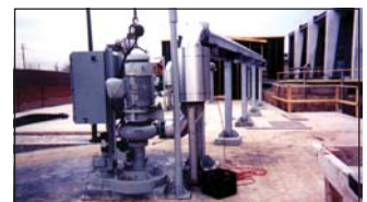
Ontario - Municipal Wastewater Complete PISTA® Grit Removal System 1,590,000 m 3 /d
